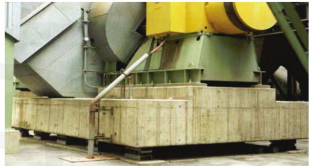
Fig. 6.3.3a—Isolator-supported fan foundation (photo courtesy of GERB Vibration Control Systems, Inc.).
