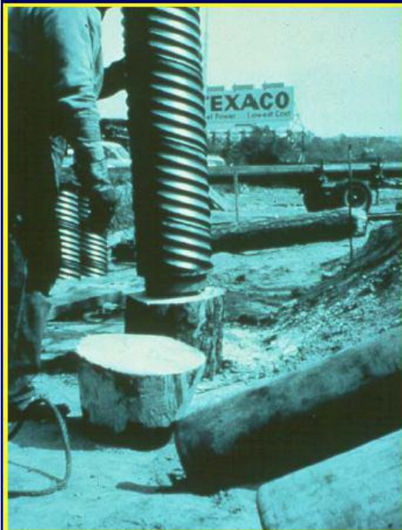
Corrugated Shell - Timber
