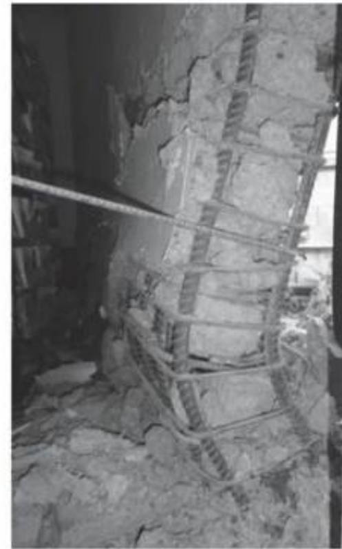
(b) 2011 Christchurch earthquake
